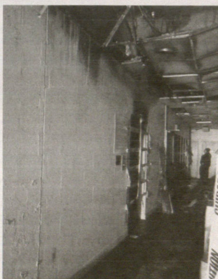
Fire Damage at Lower Level of JCC
